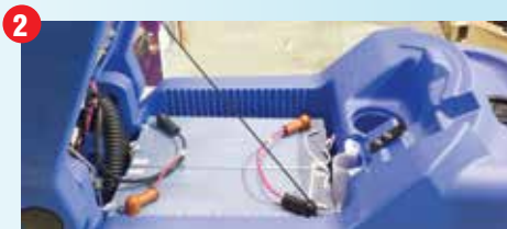
Compartment des batteries / Battery compartment
